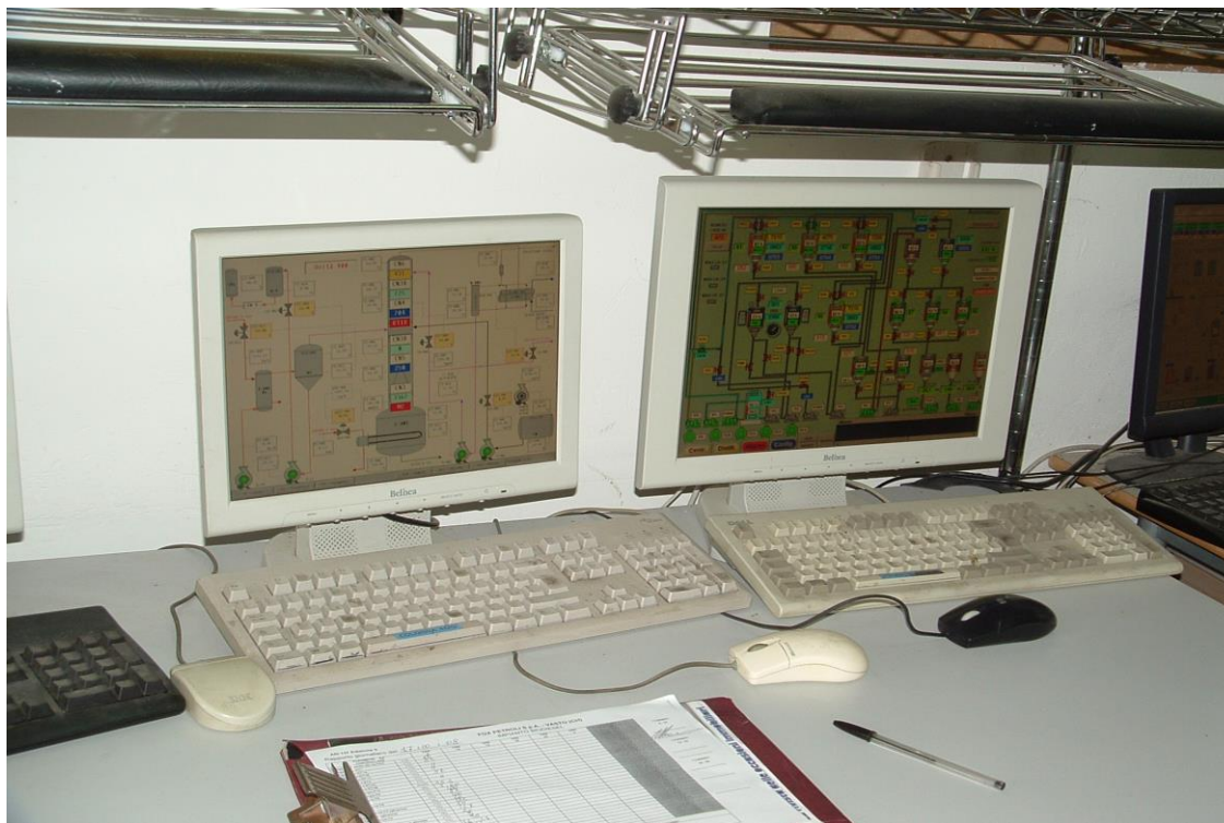
The Biodiesel plant Control Room. The plant workers can control the whole process using the redundant Movicon supervision workstations.
