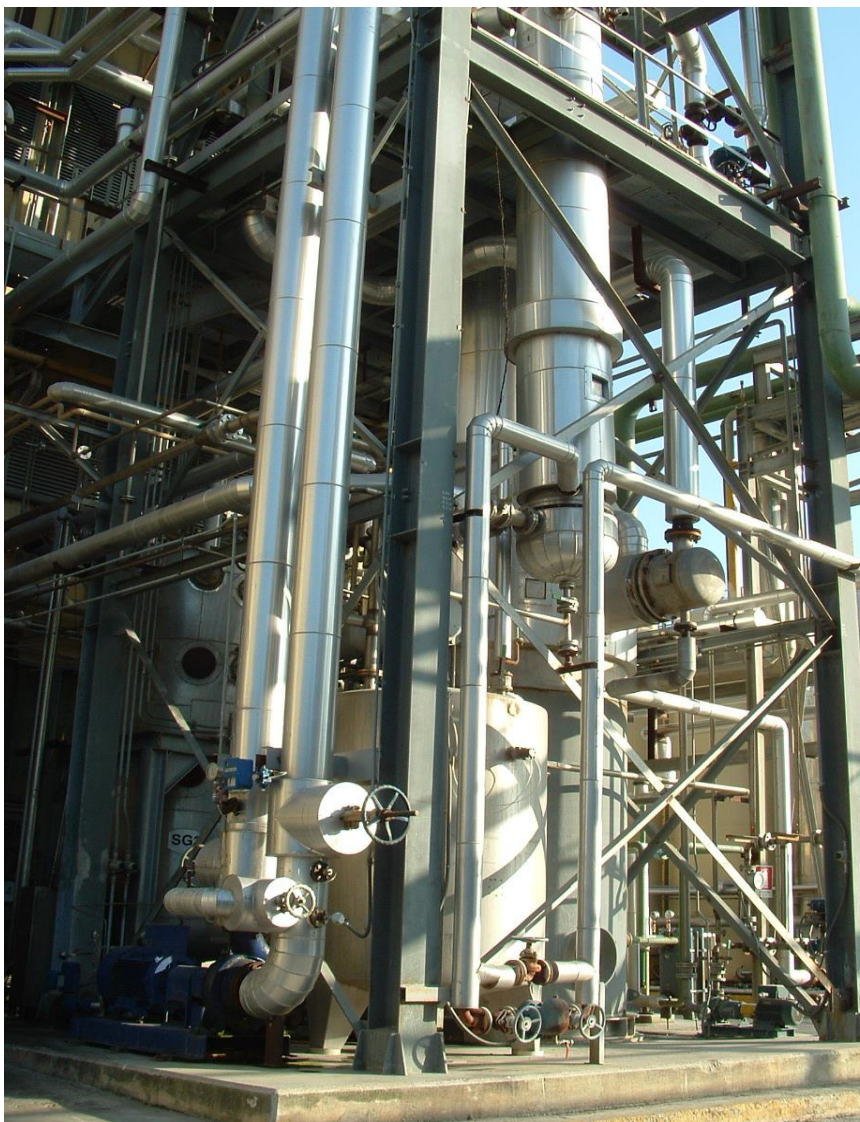
The revamped Fox Petroli biodiesel production plant.
